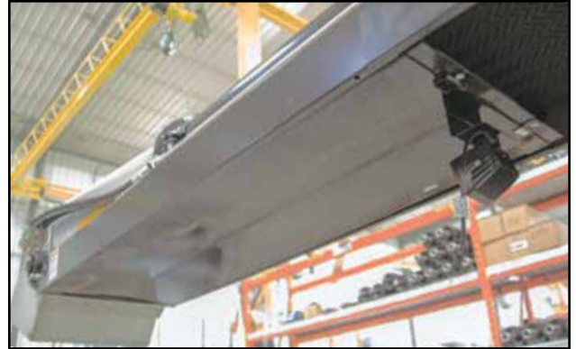
Fig 12 - Discharge Drip Pan
